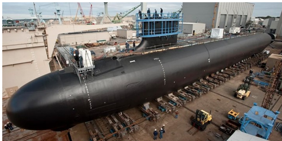
The Columbia-class ballistic missile submarine USS District Of Columbia (SSBN 826), under construction.
