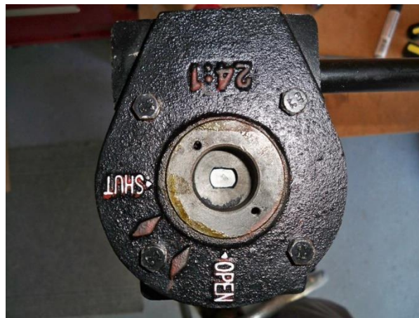
FIGURE 12 (Position indicator cover removed showing valve in CLOSED position)
